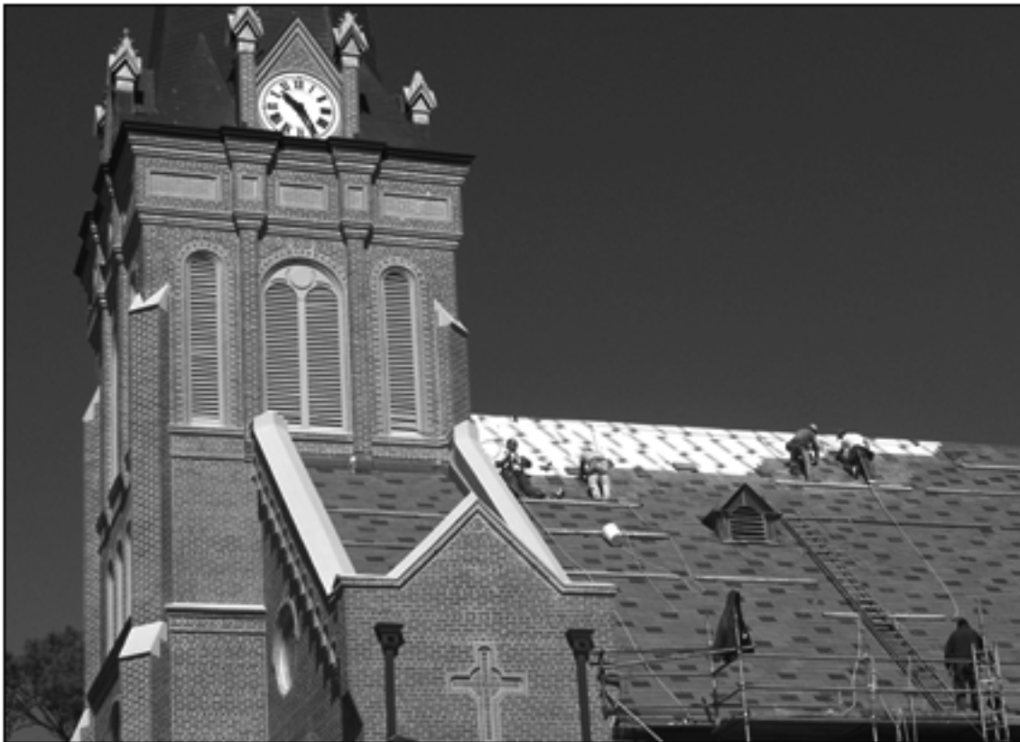
The Rectory side of church nears completion as workers lay the slate tile in a random color pattern.
